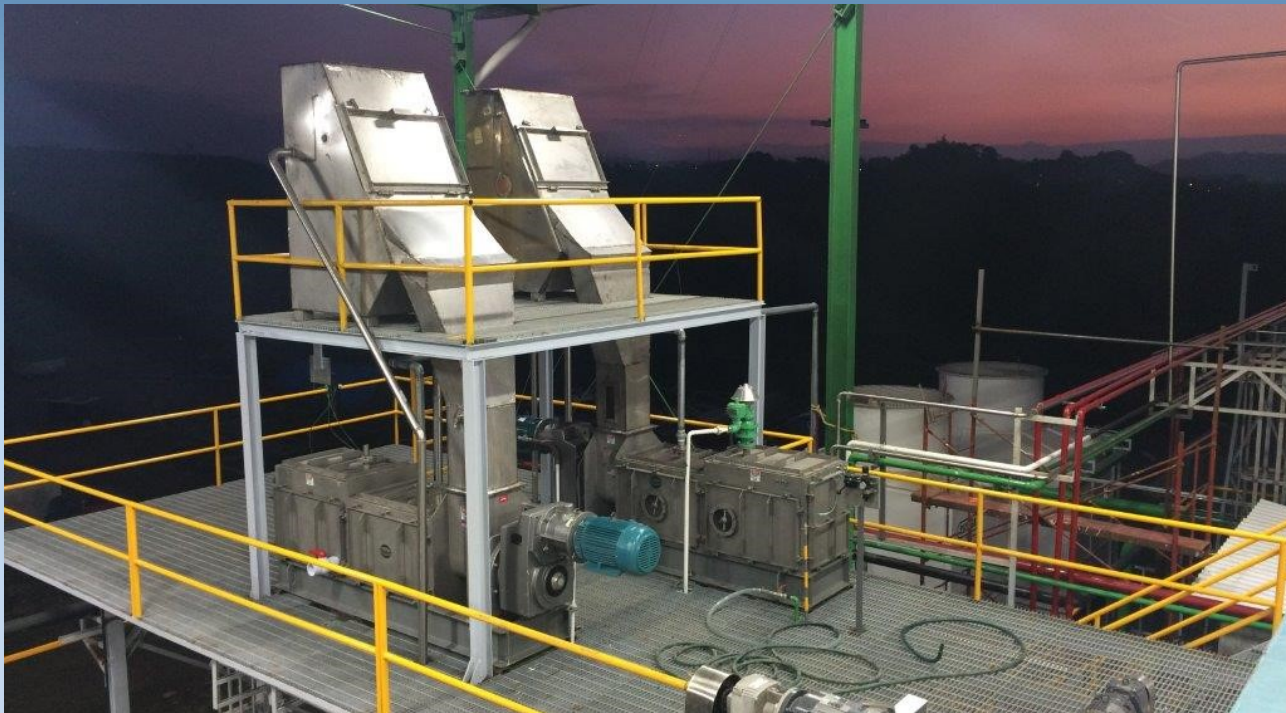
Pair of Vapor Tight KP-12VT Presses
