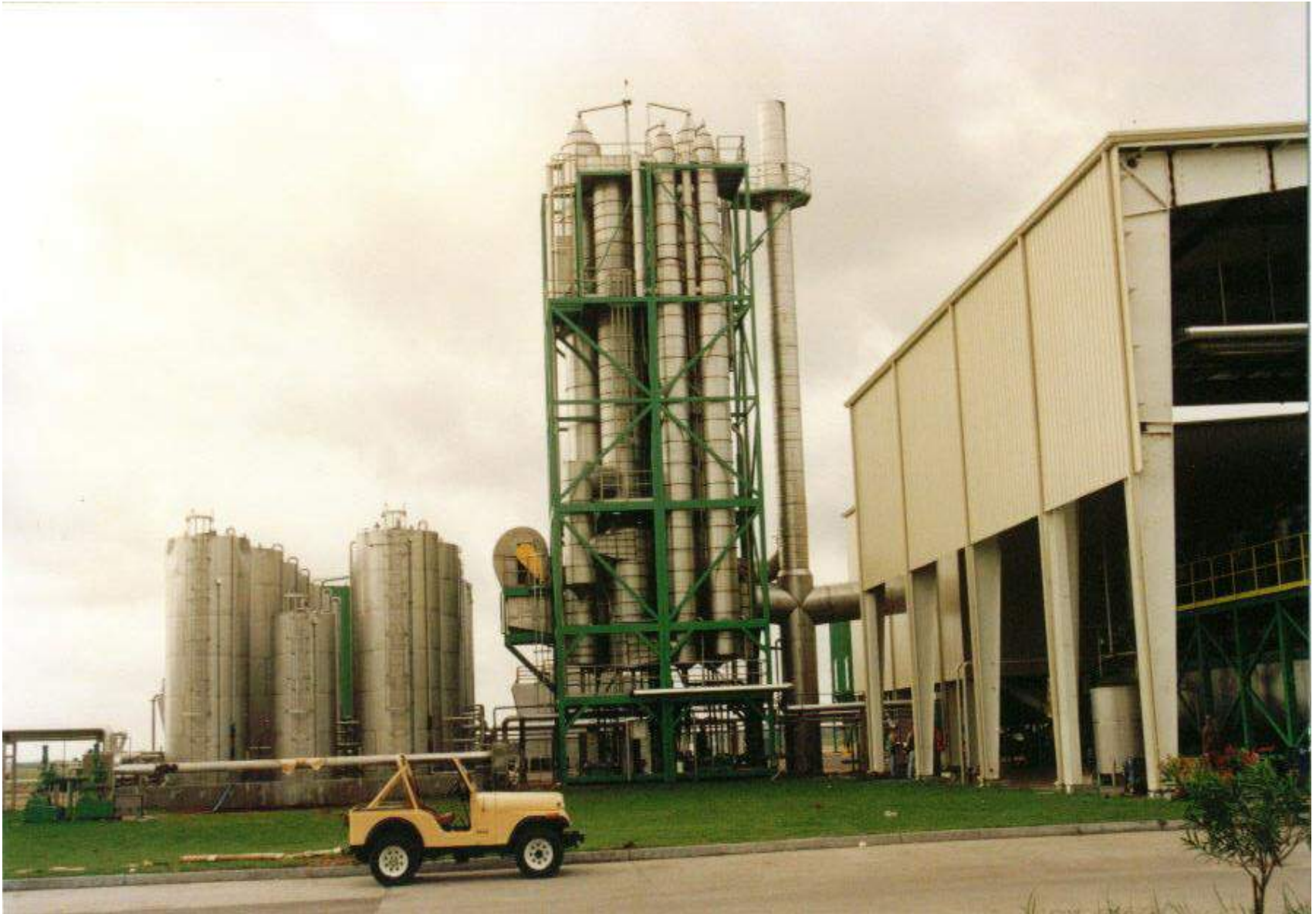
Figure 7: Waste Heat Evaporator
